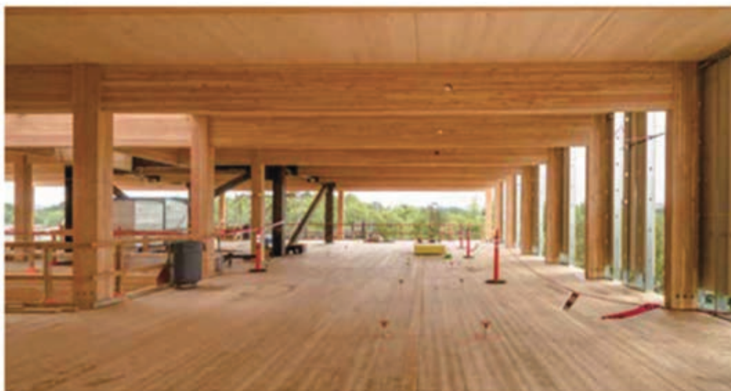
FIGURE 6.4: A CLT AND GLULAM MASS TIMBER OFFICE BUILDING First Tech Federal Credit Union, Hillsboro, Oregon; Source: Swinerton Builders
